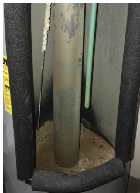
A look inside a water heater that has reached the end of its service life with 3 inches of sediment at the bottom.
